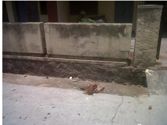
View of ground floor of Wilson Garden quarters (water level goes up to red mark)
