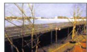
Fall Protection Fence
