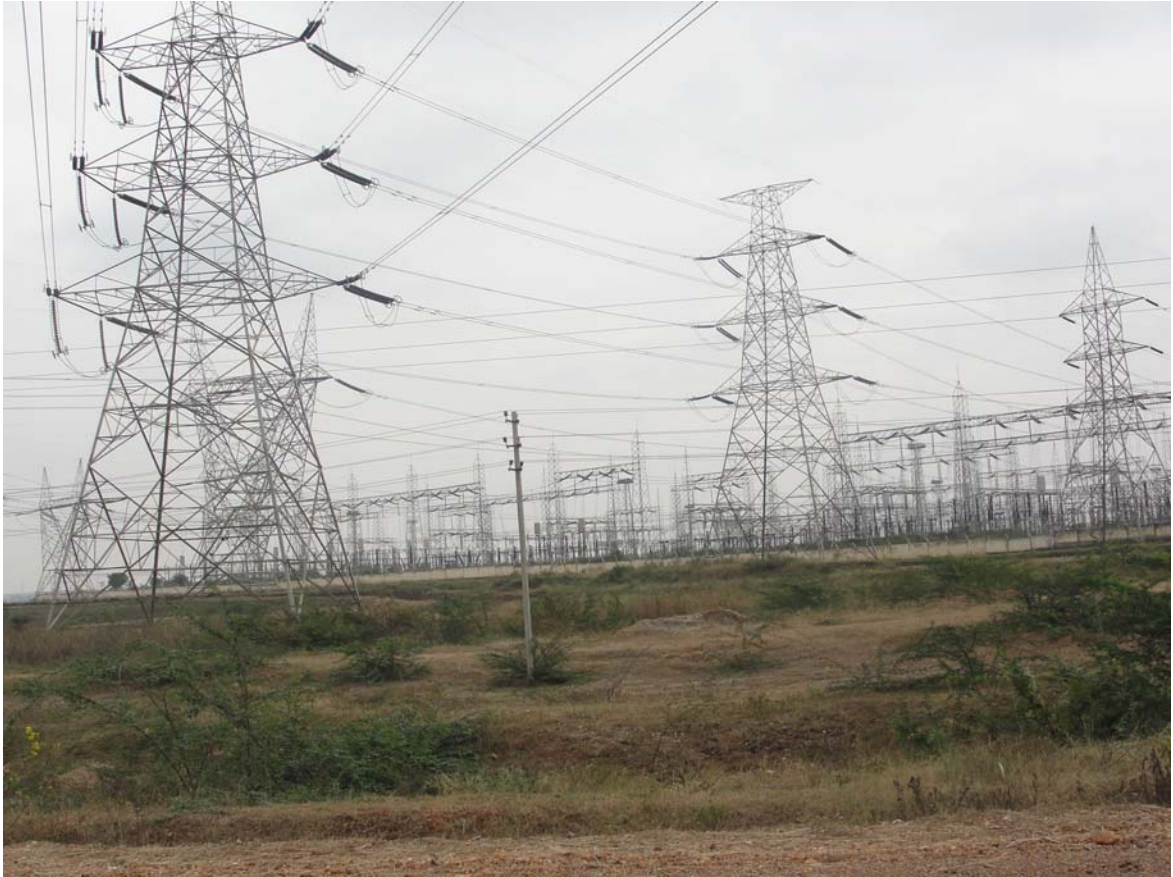
Fig 3.5: A snapshot of Guttur Sub-station
